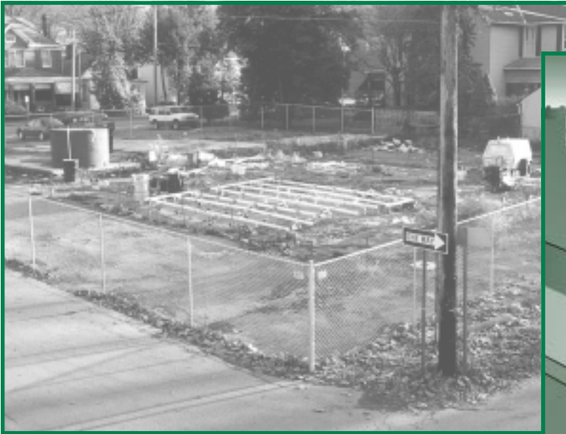
A pilot-scale test of the Well Injection Depth Extraction system was conducted at an abandoned gas station in Weston, WV. The system effectively removed chemical contaminants that were threatening the nearby West Fork River.
